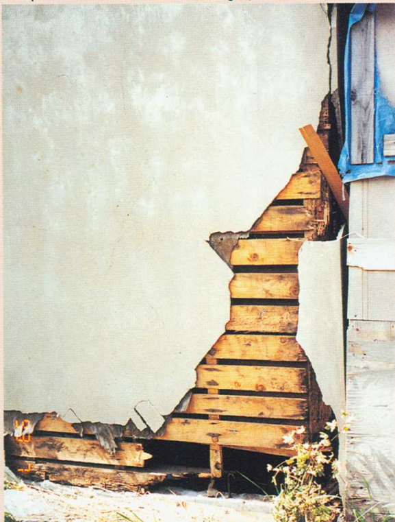
Fire preventive construction flaming up due to fire brands
