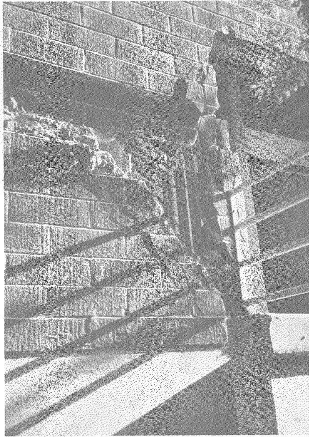
Fig. 41 Diagonal cracking and crushing of heavily reinforced masonry.
