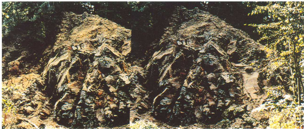
Photo 6 Basalt rock that appeared on a failure surface
