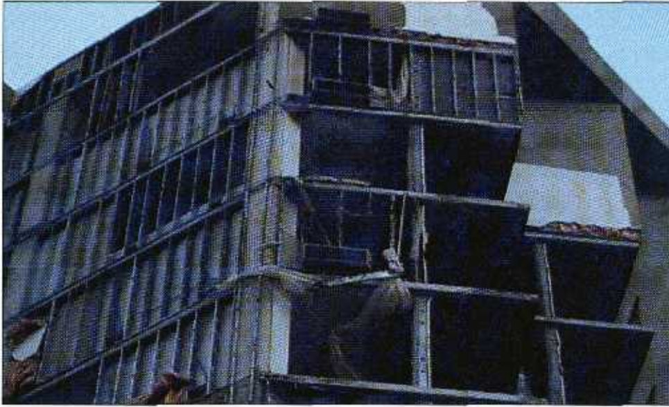
FIGURE 5-7 This EIFS wall system was composed of synthetic stucco over 1-in thick expanded polystyrene insulation (EPS) over a layer of exterior gypsum board over 6-in deep steel studs, with a layer of gypsum board on the interior side of the studs. Fiberglass batt insulation was installed within the stud cavity. There were several different planes of failure. Insufficiently attached stud tracks appeared to have been the initial failure point. This building was located on Isla Verde.
