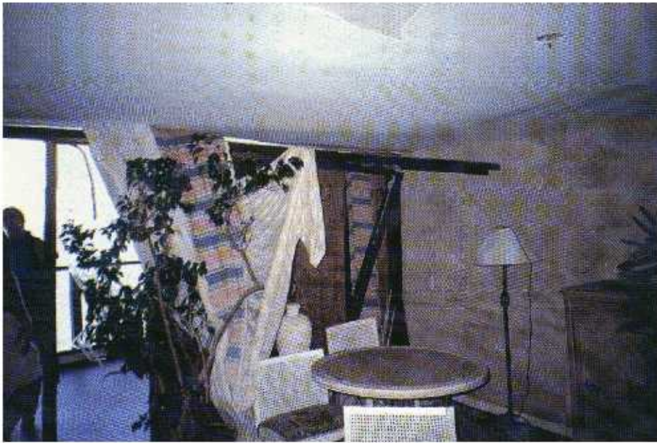
FIGURE 5-1 This sliding glass door and window assembly in a hotel room was 7' 2" high and 14' long. The head of the frame was attached with four pairs of #12 or #14 screws in plastic sleeves. The sleeves pulled out and the entire length of the frame was pushed inward, resulting in substantial glass breakage. This building was located on Isla Verde in San Juan.
