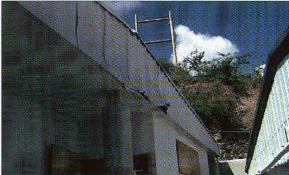
FIGURE 5-6 Rain entered this hospital on Culebra after a water tank struck the metal wall panels.
