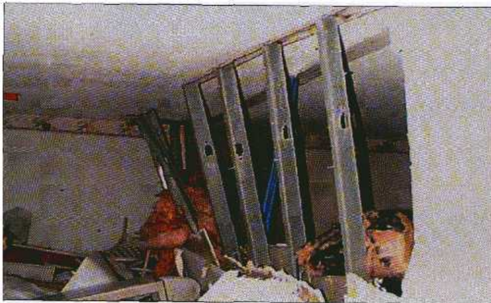
FIGURE 5-5 The gypsum wallboard was blown off this interior partition after the exterior non-load bearing wall was blown away, allowing an uncontrolled, rapid increase in internal air pressure.
