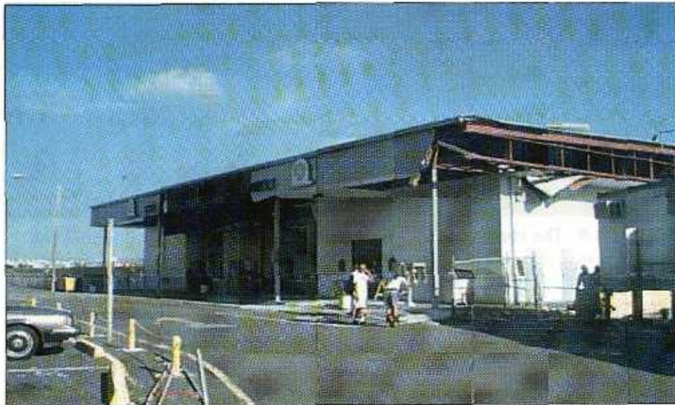
FIGURE 5-8 Several composite panels blew off from the fascia and soffit of this building at the airport on Isla Grande. Although several screws were installed, the metal into which they were driven was too thin to develop sufficient blow-off resistance to withstand the wind loads.
