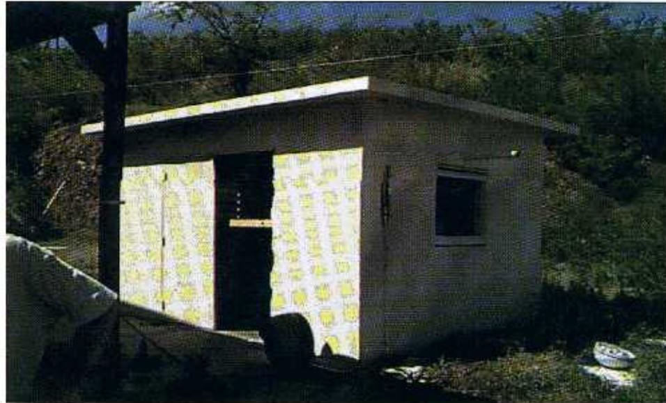
FIGURE 5-3 A missile traveling right to left struck the window louver. The door frame was attached by fasteners into wooden plugs that had been set into holes drilled into concrete. Once the louver failed, the door frame failed.
