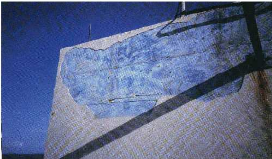
FIGURE 5-9 The stucco was blown off the corner area of this wall, where the suction pressures were high. Note the rough texture of the concrete.
