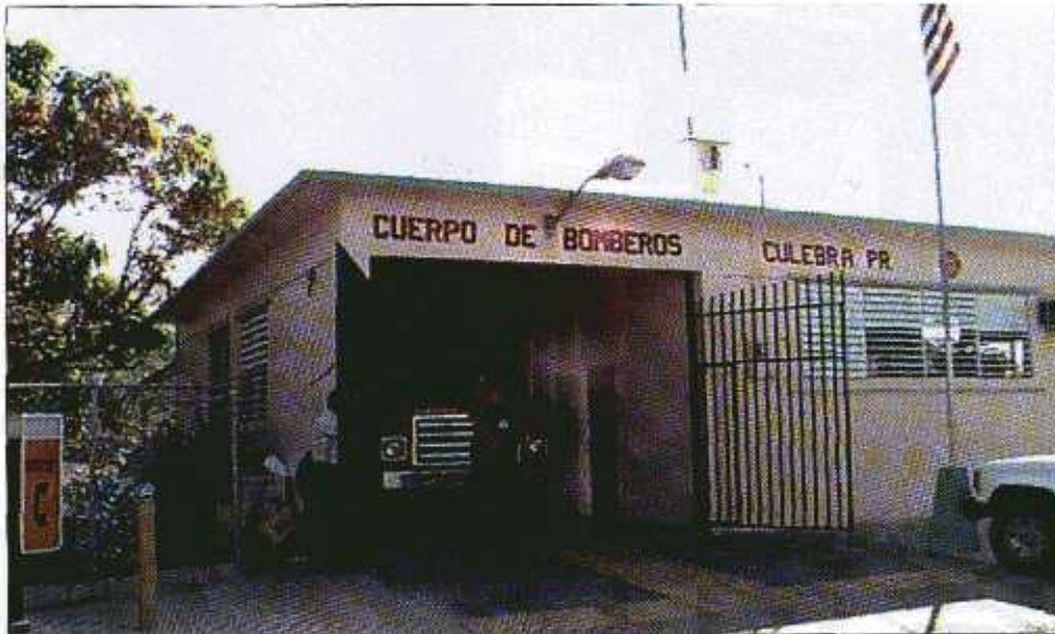
FIGURE 5-4 The security grille on this fire station offers greater wind performance reliability than a solid door because very little air pressure is applied to it during high winds. This fire station is located on the island of Culebra.
