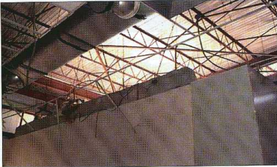
FIGURE 5-41 Part of the exterior envelope of this building blew away, resulting in damage to the acoustical ceiling. This revealed a lack of seismic resistance of the ceiling system, light fixtures, and ductwork.
