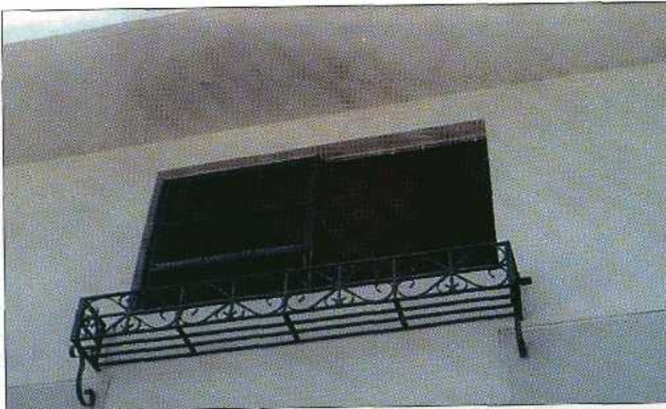
FIGURE 5-26 Half of the window frame blew out. It was attached with two screws in plastic sleeves at the head, three screws at the jamb, and two screws at the sill.
