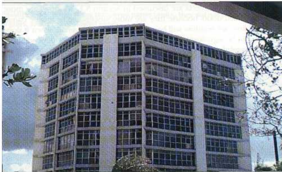
FIGURE 5-23 The windows in this building were broken by aggregate from the built-up roof of a nearby building (Figures 5-24 and 5-25).
