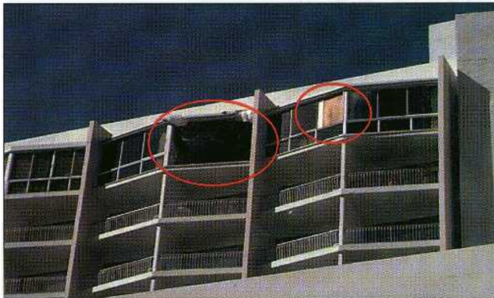
FIGURE 5-29 The glass and frames were blown out at the center room on the top floor. At the room to the right, one of the glass panes was blown out.
