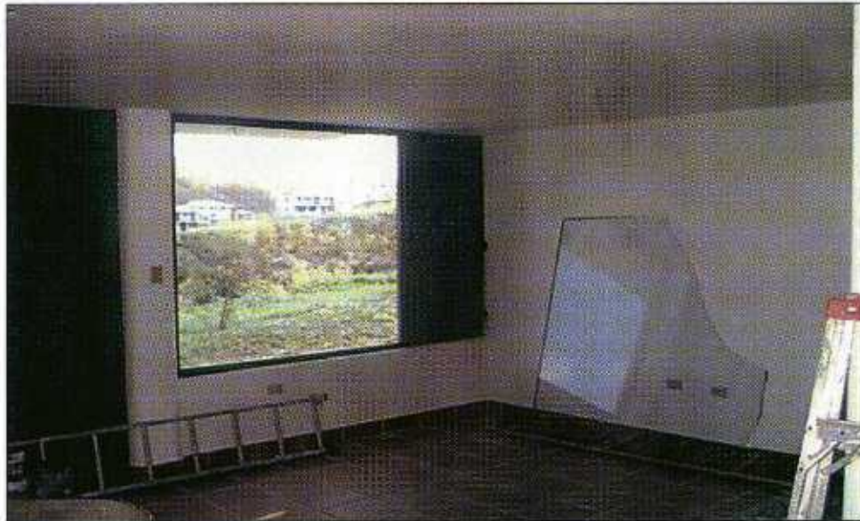
FIGURE 5-28 This large window, which was removed and leaned against the wall after the storm, was broken by a missile, most likely a tree limb.
