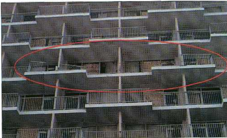
FIGURE 5-31 High-energy missiles from a nearby building damaged several railings of this building.
