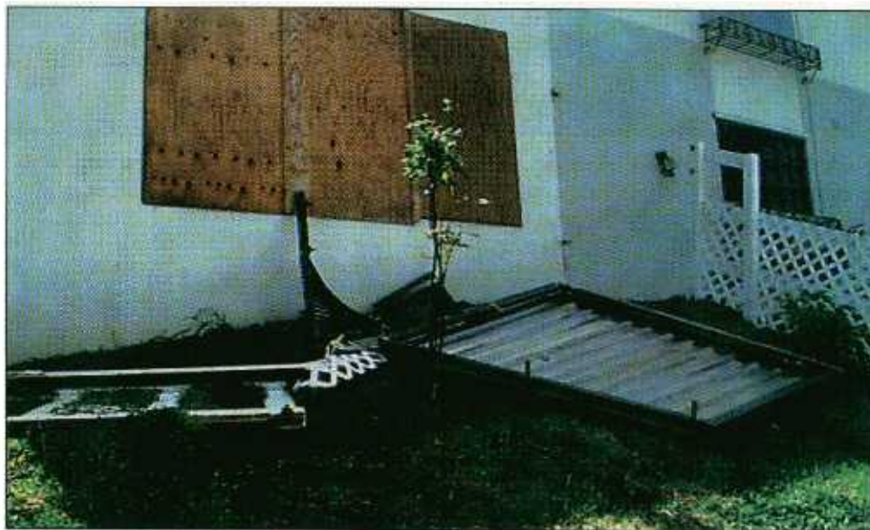
FIGURE 5-40 The window lying on the ground was protected by a shutter. However, the shutter was attached to the window frame. The window frame fasteners were over-stressed and the entire assembly failed. Attachment of the shutter directly to the wall framing is a more reliable method of attachment.
