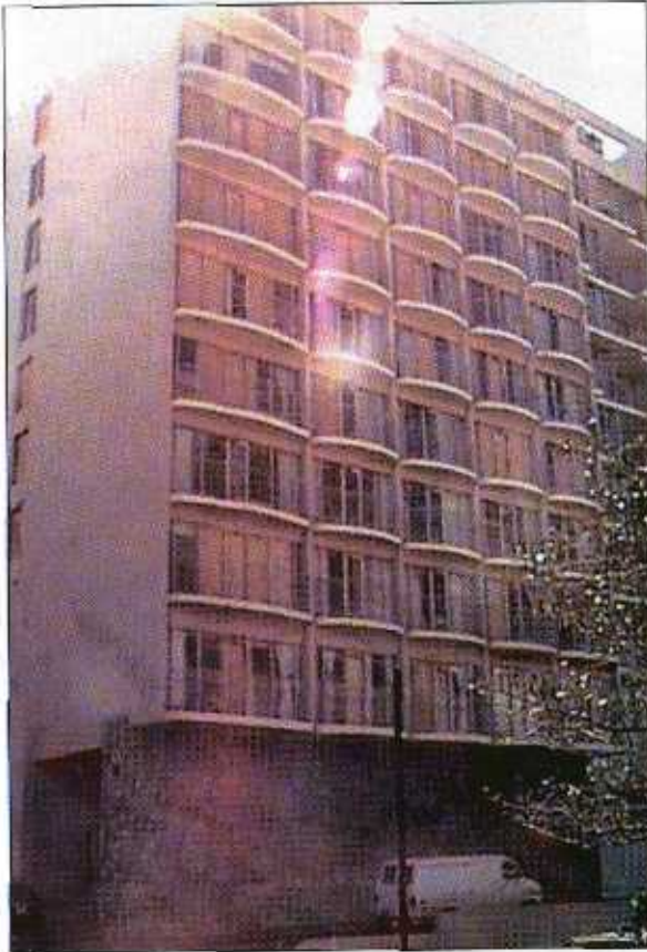
FIGURE 5-30 Several window and glass door openings broke during the hurricane. They were subsequently covered with plywood (Figure 5-31).
