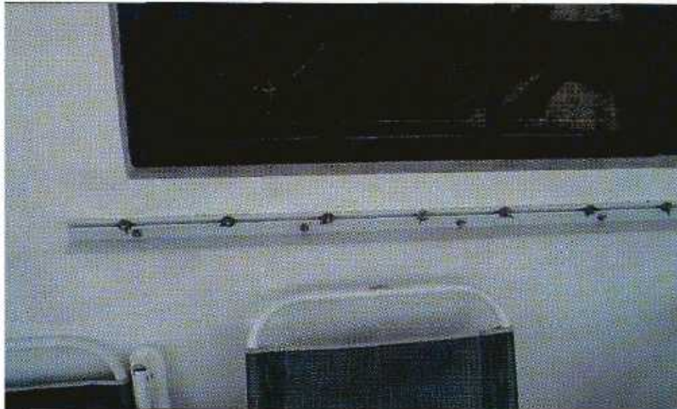
FIGURE 5-35 Close-up of Figure 5-34. The steel shutter panels were designed to be locked into the track with wing nuts spaced 6-in on center, a more reliable attachment than that shown in Figure 5-36.
