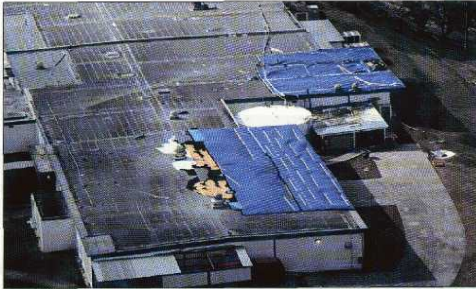
FIGURE 5-22 This built-up membrane had a mineral surface cap sheet. Because of the roof covering damage, this manufacturing facility on the island of Culebra was shut down for approximately two weeks after the hurricane. This building also experienced roof damage during Hurricane Hugo in 1989.
