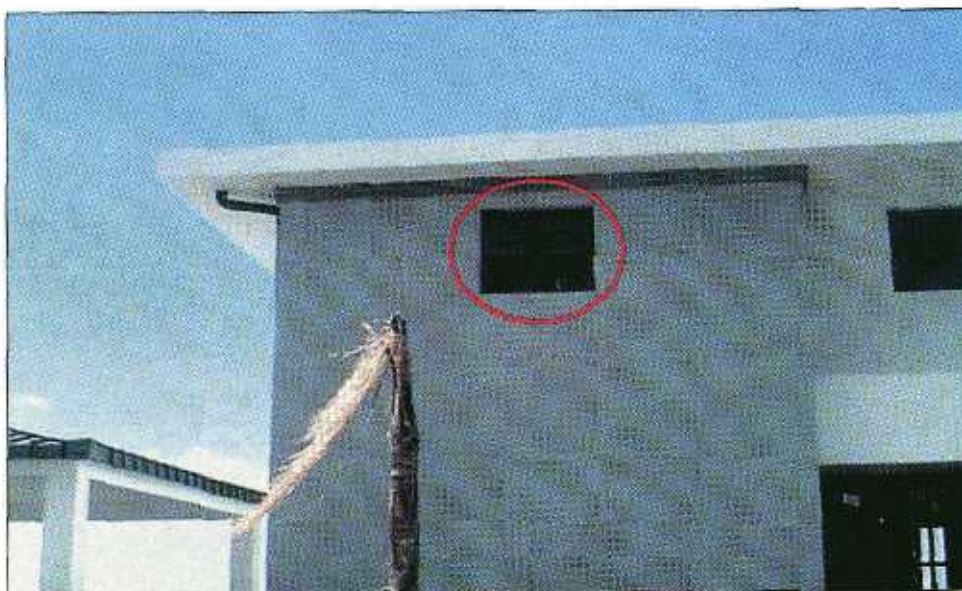
FIGURE 5-27 One pane in this window was broken by a missile, perhaps from the palm in the foreground.
