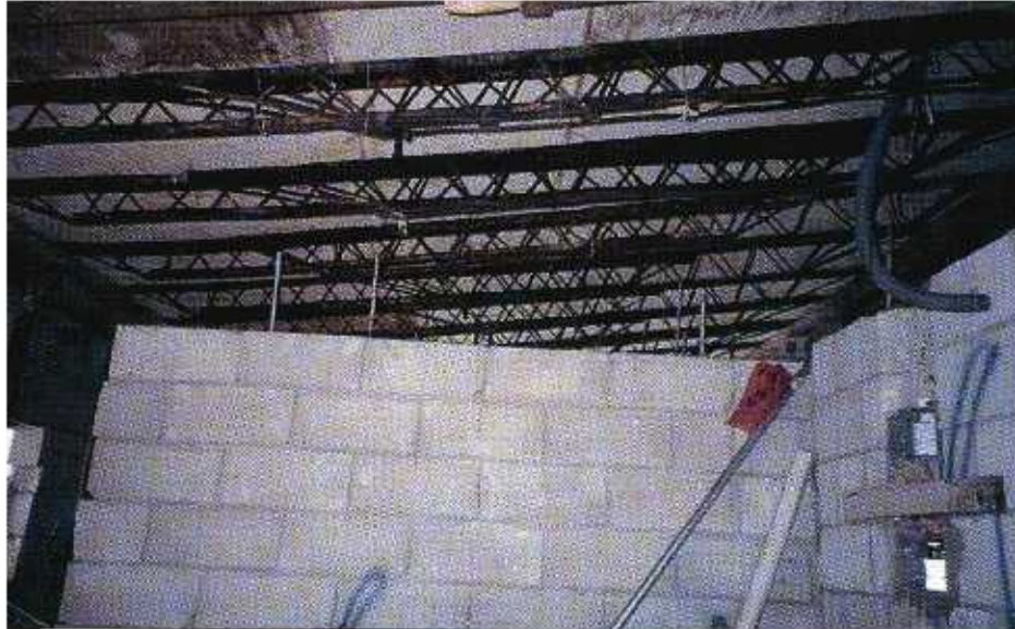
FIGURE 5-42 An interior view of a house under construction (the steel joists are supporting formwork for the concrete slab). The CMU partition is inadequately reinforced and is not supported or laterally braced at the top of the wall.
