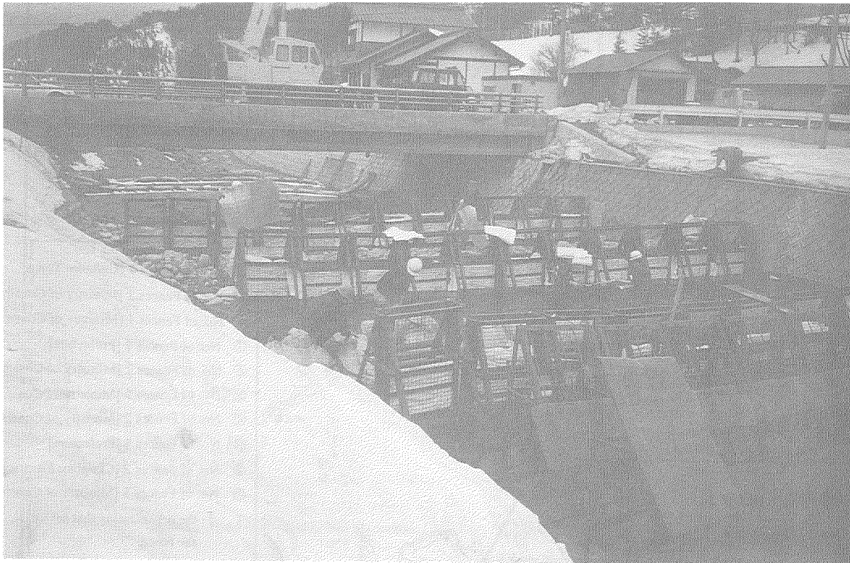
Photo 2 Setting up the river filter just upstream of the Nanmonbara Bridge (March 7)
