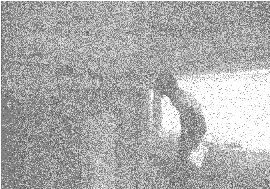
Fig. 5.6 Support of Ward Memorial Boulevard bridge deck at southern abutment. View shows piers capped by damaged rocket bearing assemblies under bridge on left in Fig. 5.5.
