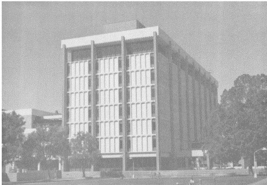
Fig. 7.38 Eight story Library III Building, UCSB. This building also sustained cracks in shear walls in lower stories.
