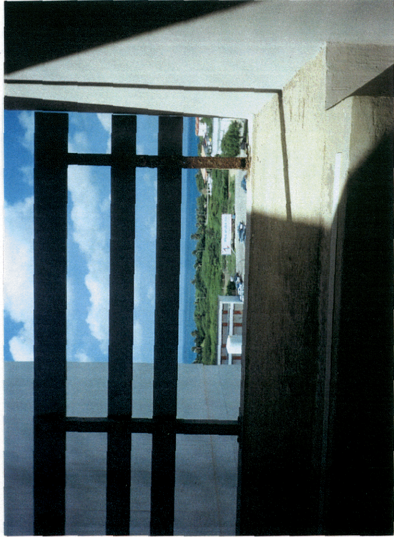
PHOTO 15 Corrosion spots on fence in the emergency stairway
