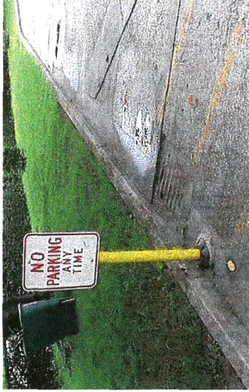
Photo 43. Car park adjacent to the South Block. The mesh in this drain is blocked with silt.
