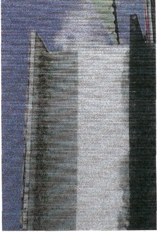
Photo 12. A long, diagonal crack at the upper North-East corner of the Physiotherapy Department. This crack continues along the East perimeter wall at the same level.
