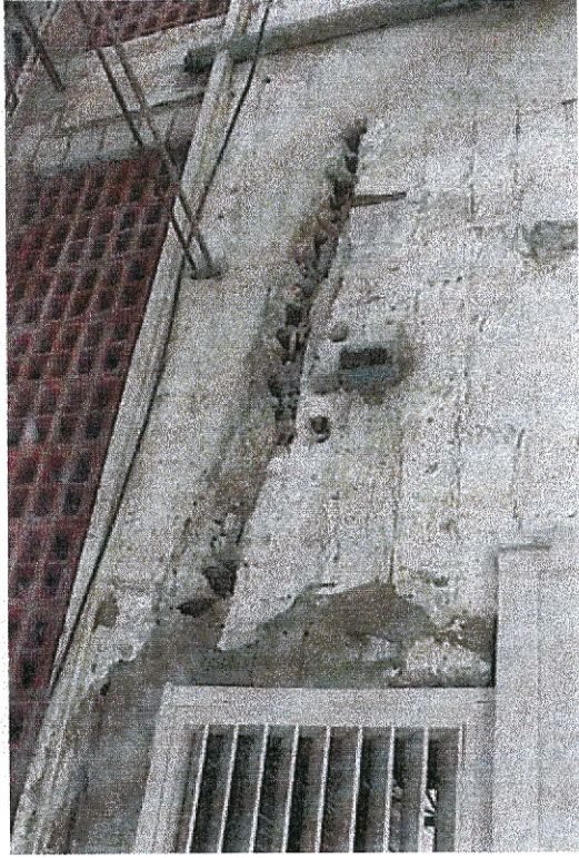
Photo 18. Extensive damage to blockwork in the East wall of the Laundry House.
