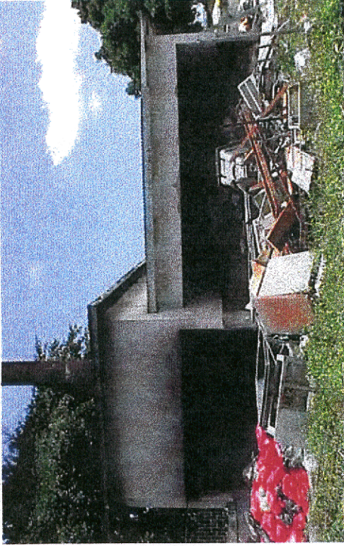
Photo 23. The harsh environment in which the Small Incinerator is located has proved to be detrimental to its condition.
