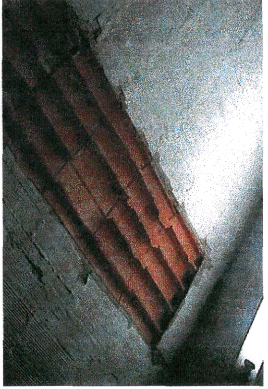
Photo 36. Damage to the soffit of an SB Slab in the South Block. The brittle nature of fired clay results in the unexpected collapse of broken portions of clay 'pots'.
