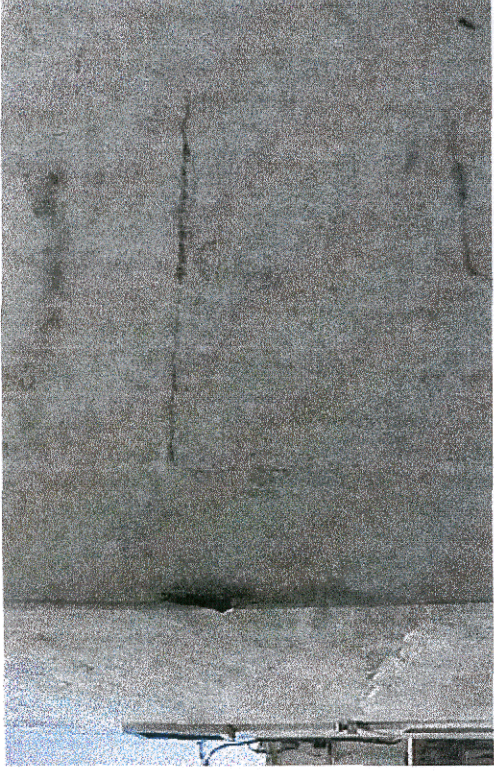
Photo 35. An example of junction cracking in the walls. The interface of structural elements and the infill clay brick wall is clearly delineated by these cracks.
