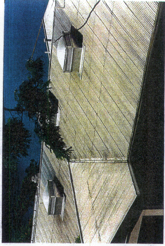
Photo 20: Roof of Psychiatric Ward. Roof vents would be more effective if located at ridge.
