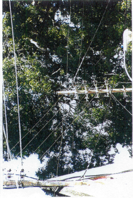
Photo 28: Electrical distribution wires suspended on poles on hospital compound. These are prone to damage during a hurricane and should be buried.
