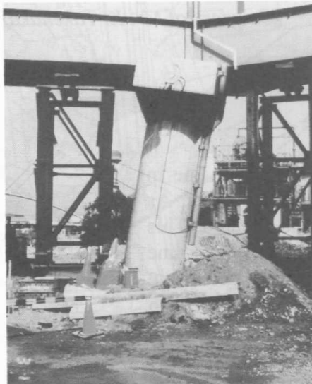
Photo 40 Inclined concrete pier due to ground displacement (A in Figure 19)
