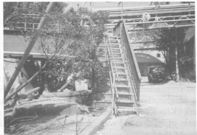
Photo 41 Separation between stairs of over-canal bridge and its concrete foundation due ground displacement toward the canal (left) (B in Figure 19)
