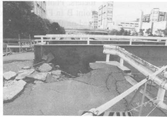
Photo 38 Movement of river bank at Ashiyahama (B in Figure 18)
