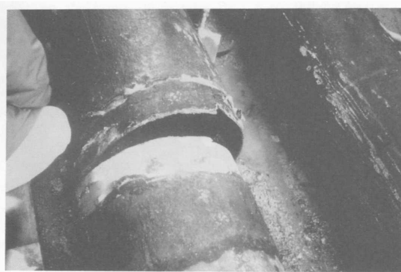
Photo 44 Rupture of welded steel water pipe (A in Figure 20)
