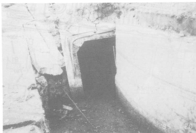
Photo 42 Floating and separation of concrete conduit due to ground displacement (Courtesy of Mr. K. Takenaka, C in Figure 19)
