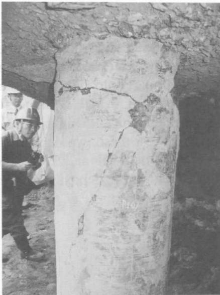
Photo 56 Failure of concrete pile on the sea side (Courtesy of Dr. H. Kiku)
