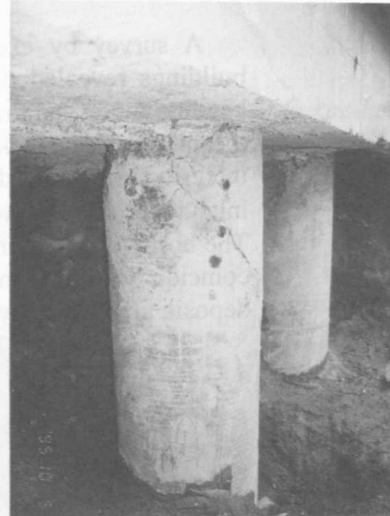
Photo 57 Cracks of concrete pile of the inland side (Courtesy of Dr. H. Kiku)
