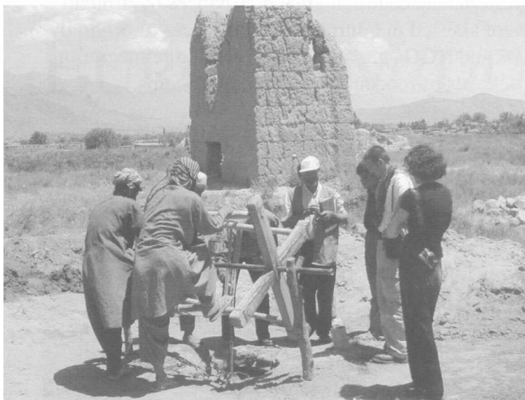
Residents of Bagram, Afghanistan constructed a well as part of a USAID/OFDA-funded water program (photo by David Plack, USAID/OFDA).
