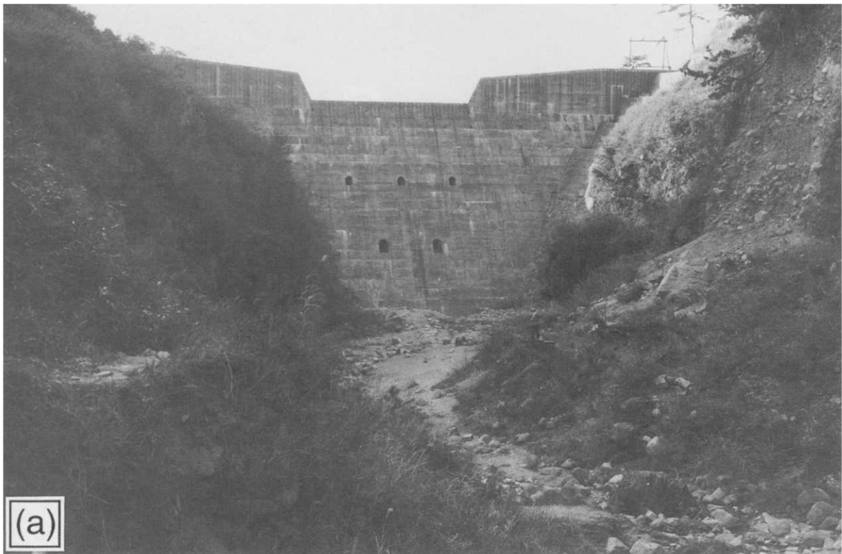
FIGURE 4 11 Gosuke check dam (height 30 m, length 78 m, storage capacity 300,000 m 3 : (a) Empty reservoir
