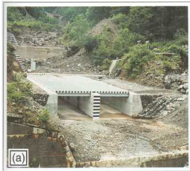
FIGURE 4.8 Debris-flow breaker in which water is drained by an iron-bar screen. (a) Before
