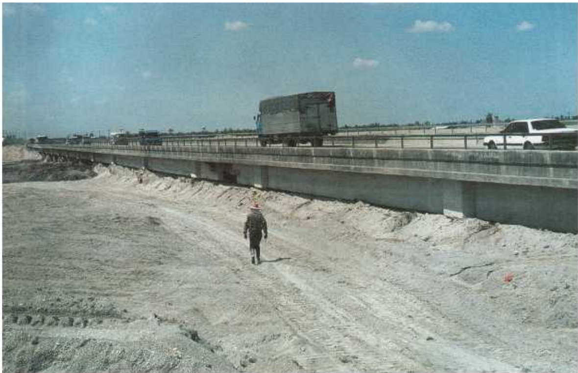
FIGURE 8.48 Upstream side of Capaya bridge over Abacan River at about km 80 from the Manila-Mabalacat Expressway. The lahar has filled the river channel up to the underside of the bridge deck. Location: Central Luzon, Philippines. Photo: R. P. Brenner, 1992.
