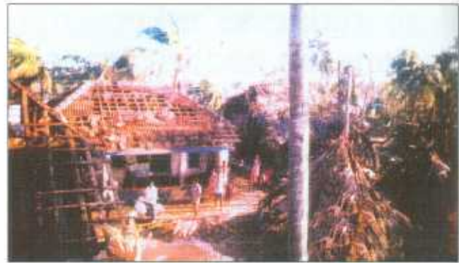
Vadapalem Village, East Godavari District : Damage to the houses due to cyclone
