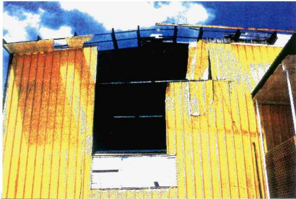
19 Crabbs Diesel Power Station - damage to gable-end sheeting
