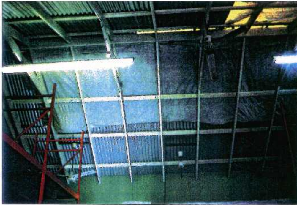
17 Friars Hill Stores - loss of roof sheeting
