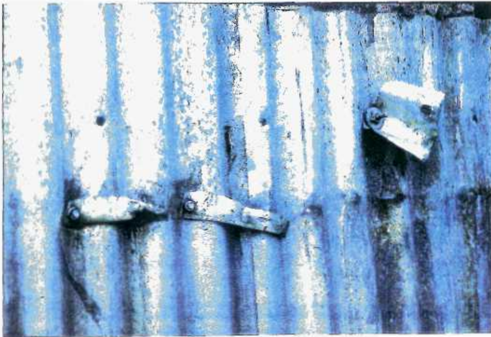
15 Friars Hill Workshop Surprisingly, the sheeting failed away from the fixing locations.
