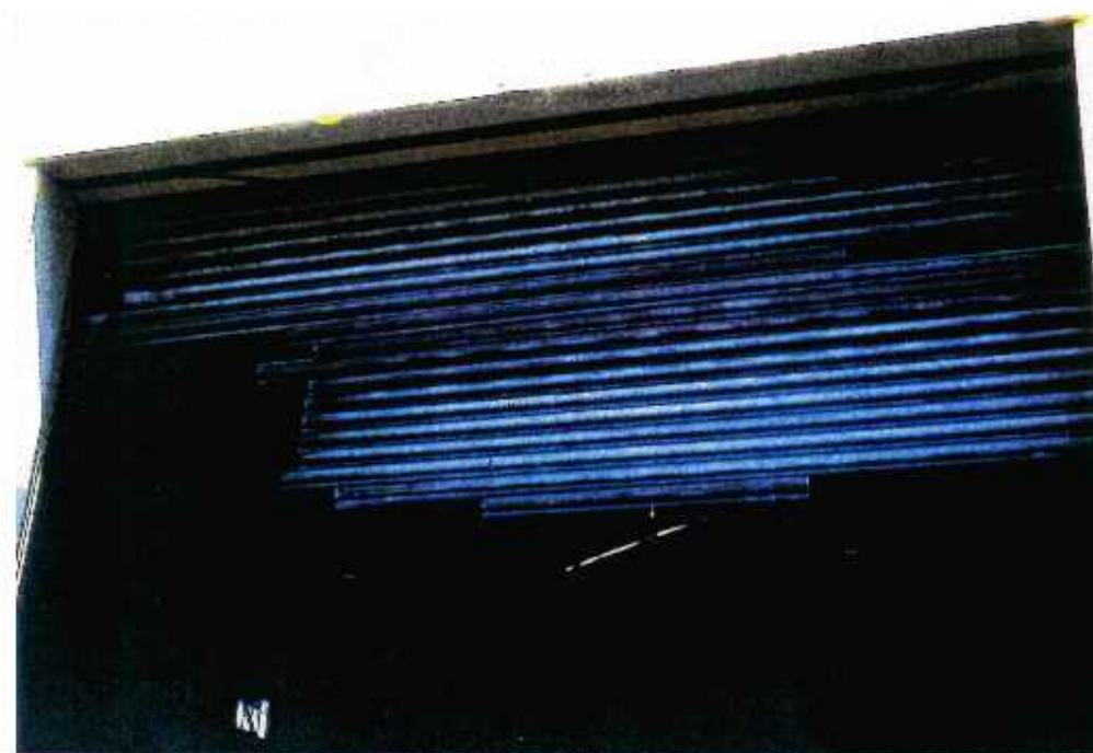
26 Crabbs Complex - destruction of roller shutter door, a common occurrence in hurricanes
