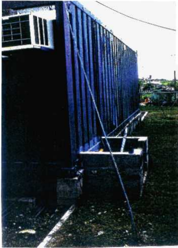
37 Swetes Substation - tie-downs were installed in advance of Luis to prevent toppling of the containers
