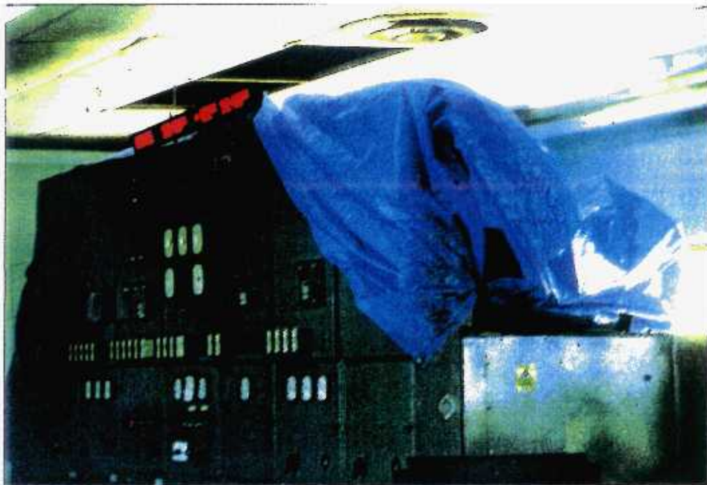
34 Crabbs Diesel Power Station - control panels were protected by tarpaulin during Luis
