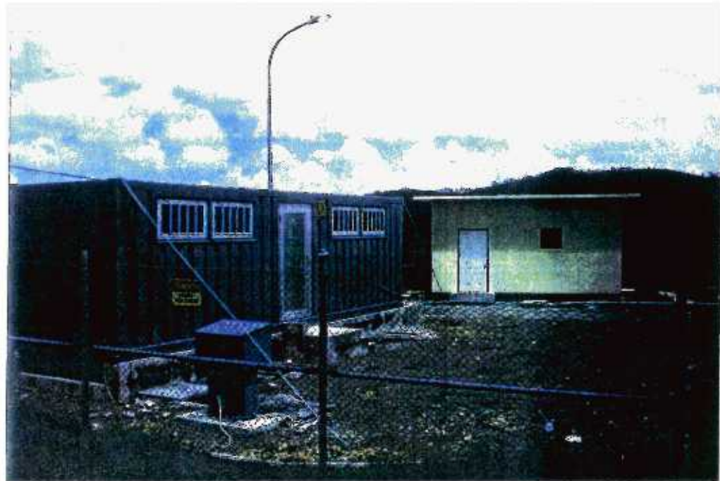
36 Belmont Substation - showing old and new types of Control Rooms
