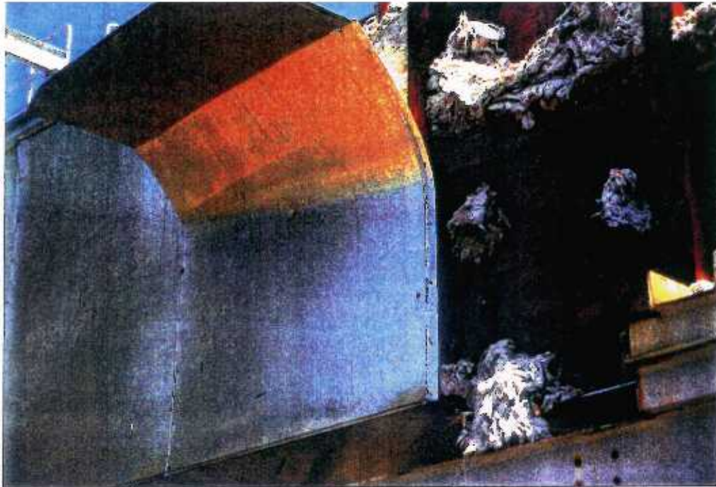
31 Crabbs Complex - close-up of damage to cladding and insulation in No 30
