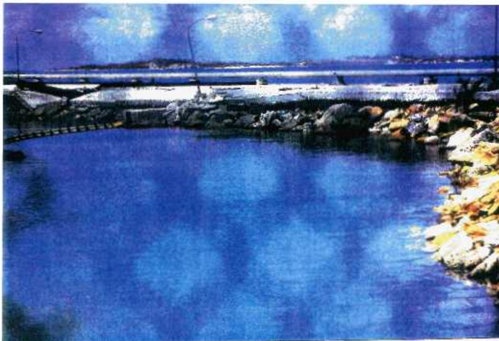
38 Crabbs Complex - destruction of marine facility at the root of the Jetty due to wave action
