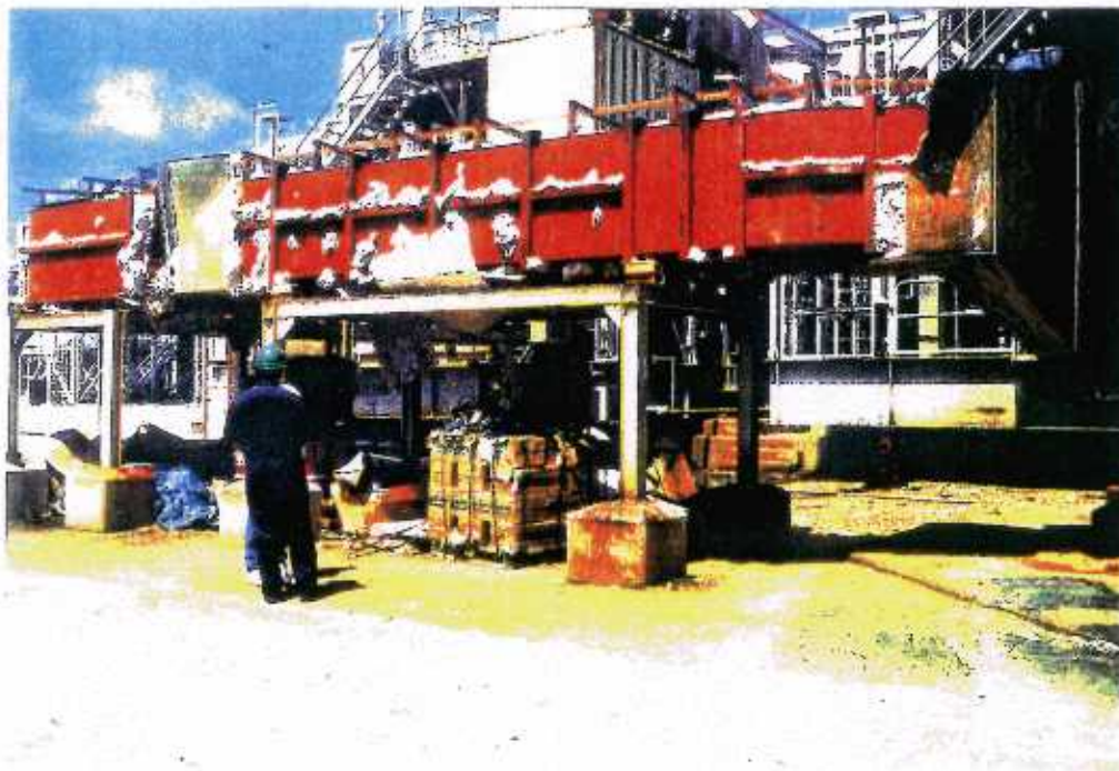
32 Crabbs Complex - damage to cladding and insulation around intake duct of Cogeneration Plant
