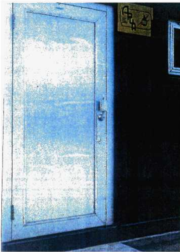
23 Typical container-type Substation Control Room showing door and window openings
