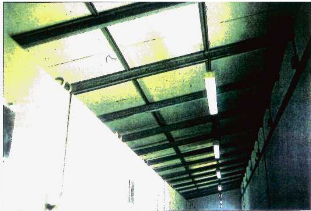
35 Cassada Gardens Complex - control panels did not need additional protection during Luis
