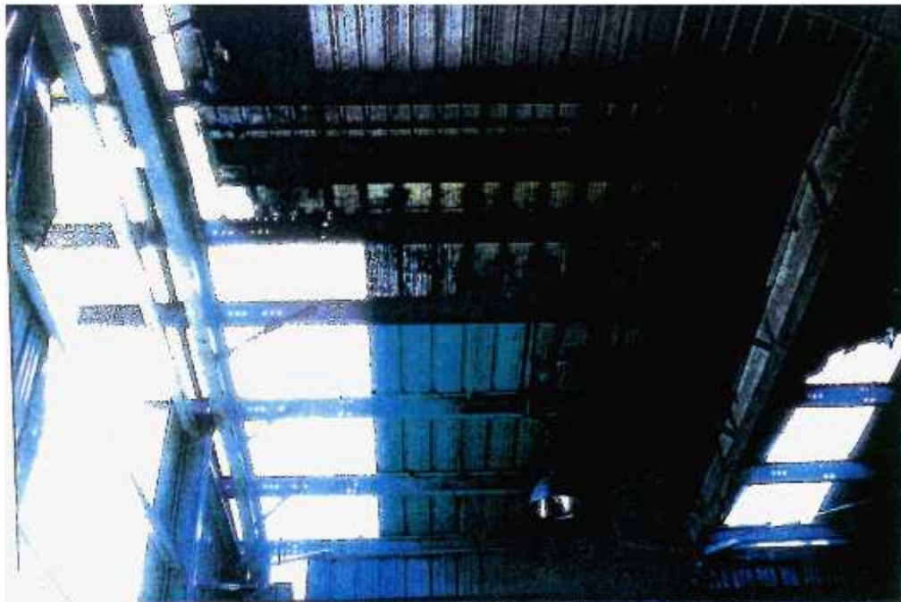
20 Crabbs Diesel Power Station - damage to gable-end wall and roof sheeting
