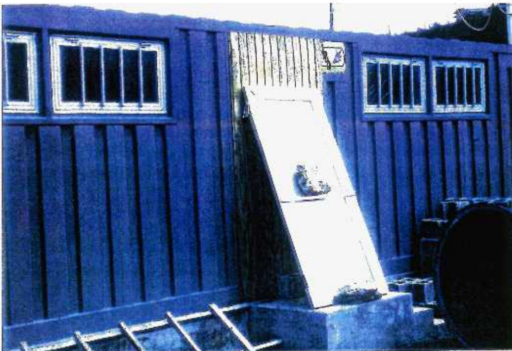
24 Typical container-type Substation Control Room showing door removed by the wind
