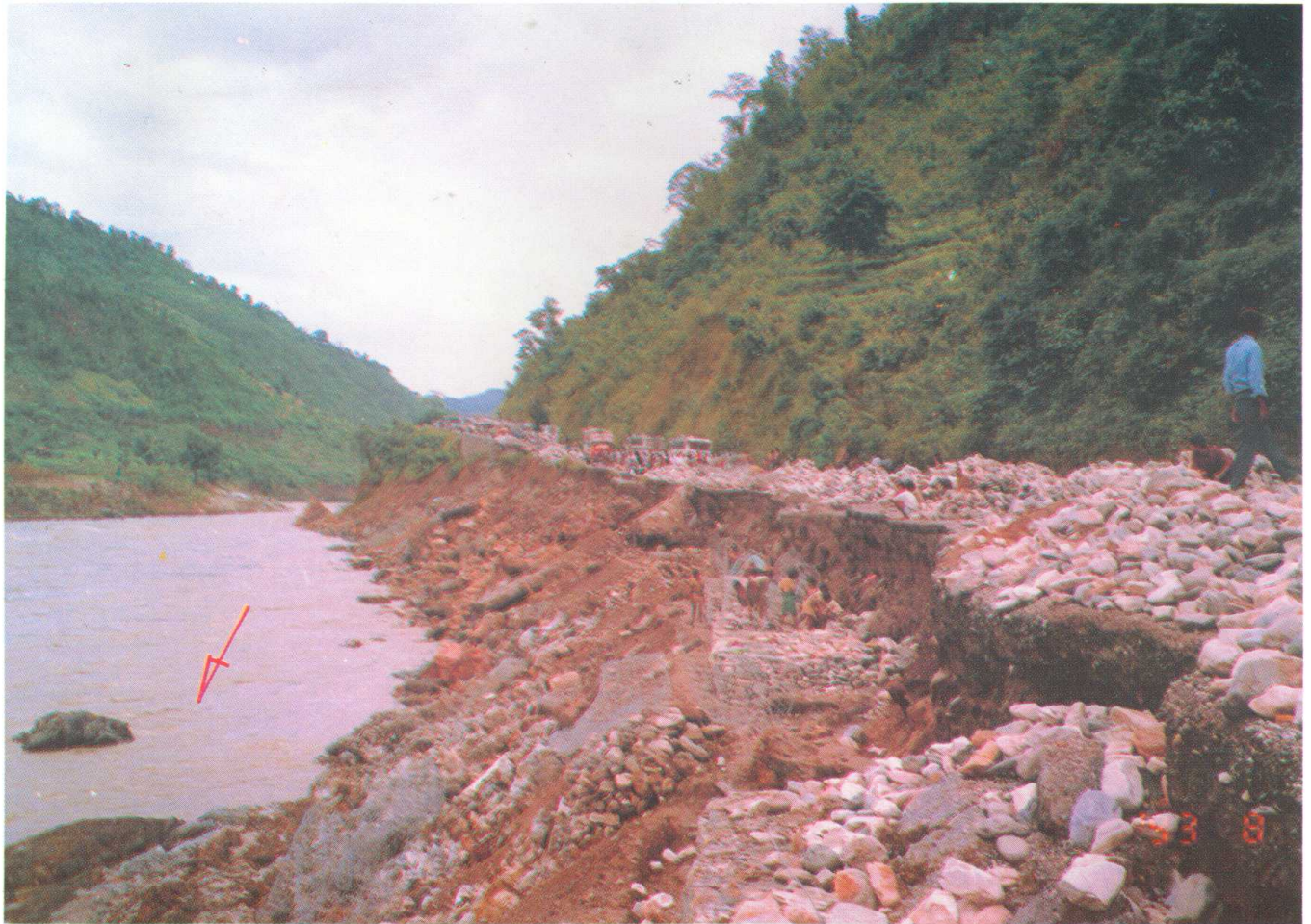
Construction of retaining walls at damaged portion of road along Prithvi Highway near Jogimara. The damage was due to bank cutting by Trisuli River.
