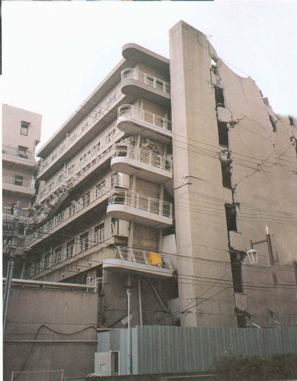
▲Damage at a hospital. Fifteen hospitals were destroyed or partially damaged.
