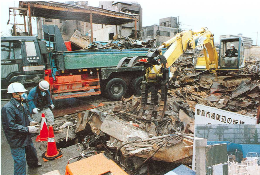
▲ Dusts emerged from collapsed buildings.
