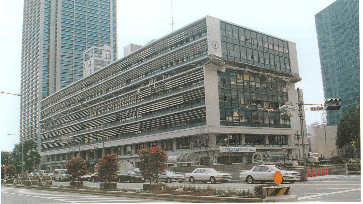
▲The Kobe municipal office building whose sixth floor was collapsed. There were some other buildings whose certain floors were destroyed.
