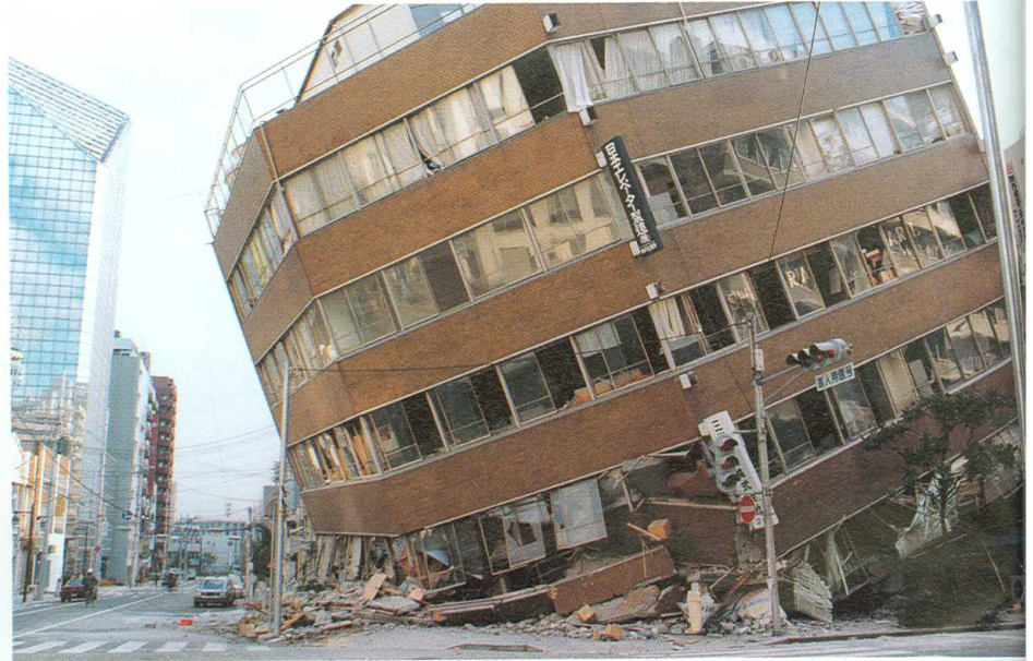
▲ A damaged building. The first floor was crushed. Damage like this was observed in most buildings with fewer walls on the first floor, such as parking places and shops.
