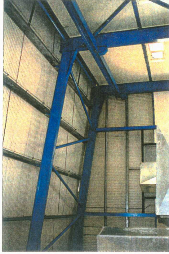
Photo 12: View of inside, Sub-station
