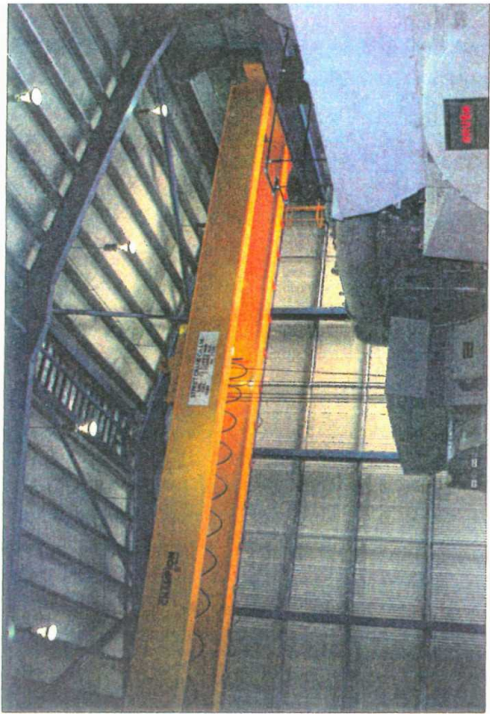
Photo 18: Power Station, internal view
