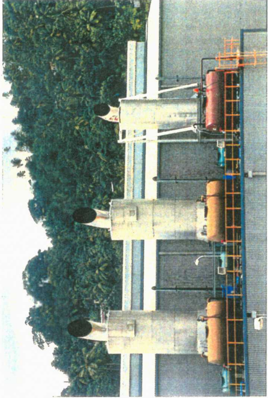
Photo 23: Power Station exhaust stacks
