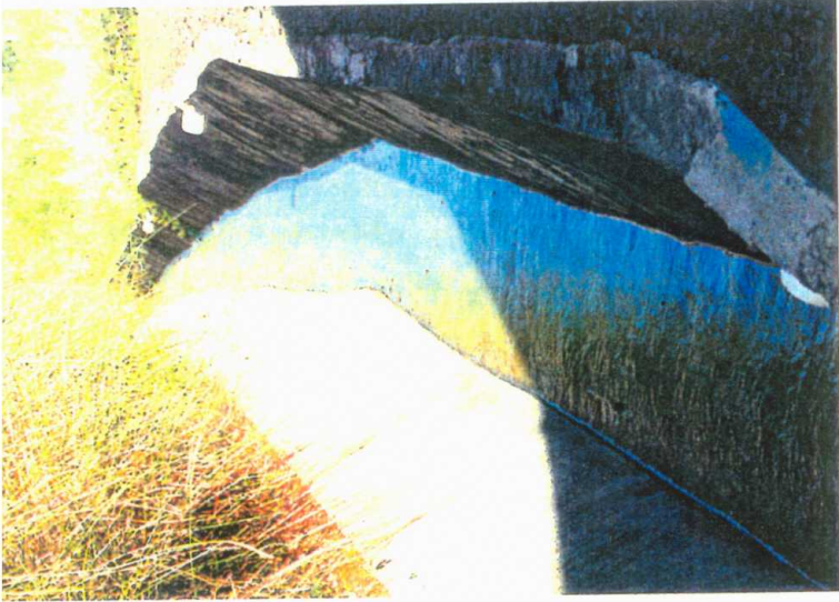
Photo 16: Main storm drain along south of site
