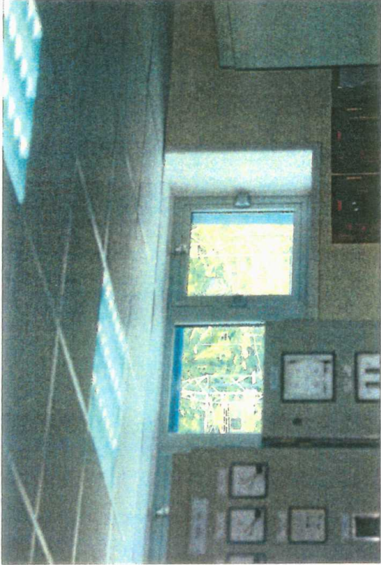
Photo 22: Power Station control room
