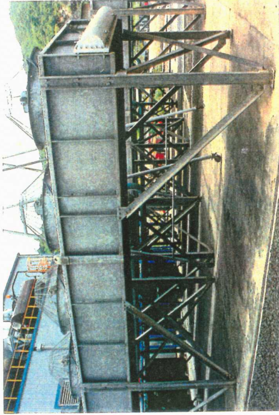
Photo 28: Radiator supports, Power Station
