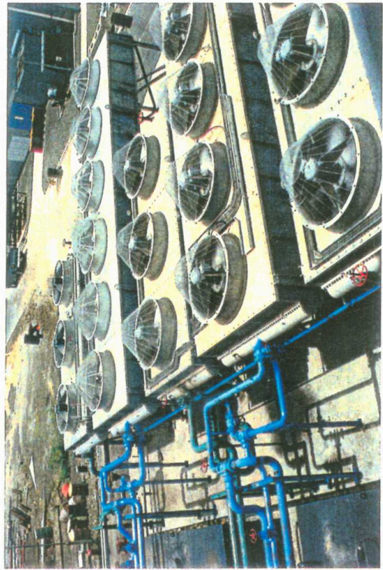
Photo 27: Radiators and connecting pipes, Power Station
