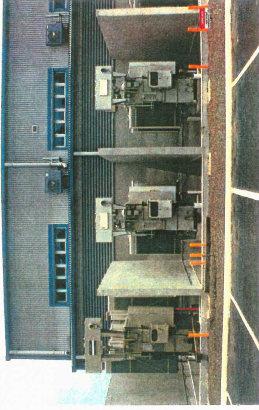
Photo 30: Transformers, Power Station
