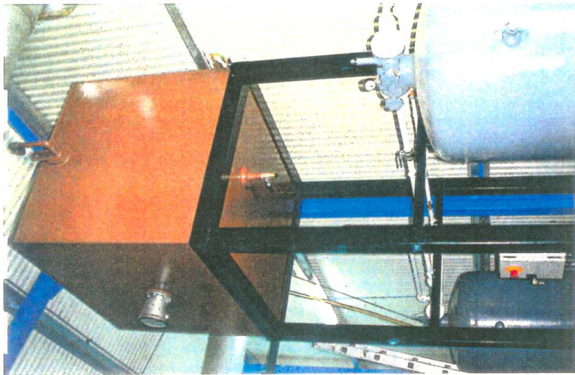
Photo 34: Typical fuel tank, Peak Lopping Station
