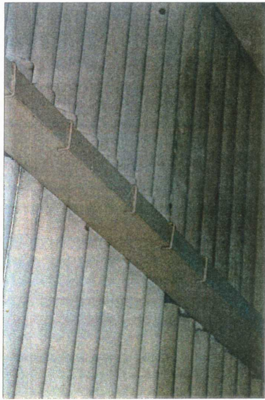
Photo 63: View of J-bolt fixing to show end which may straighten out
