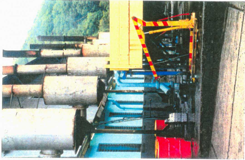
Photo 65: Power Station Exhaust Stacks
