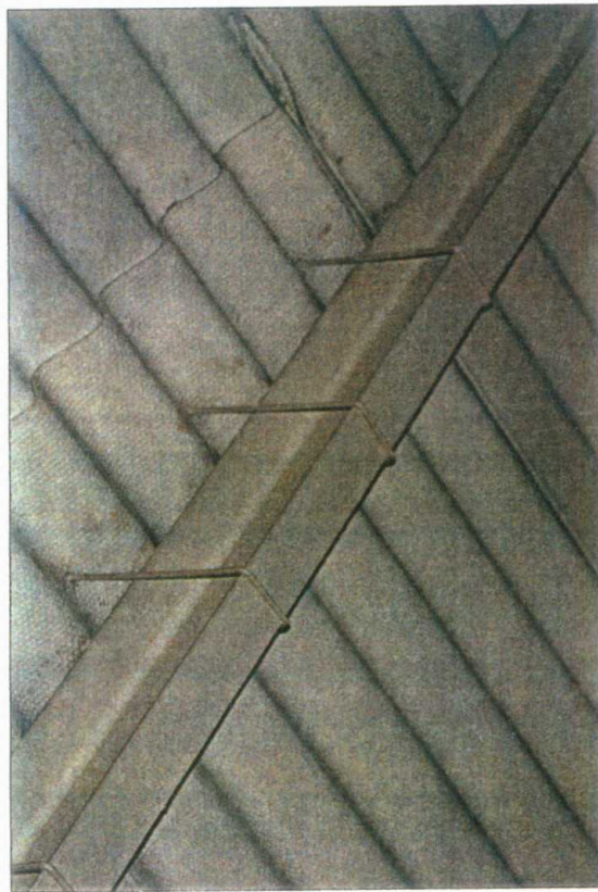
Photo 62: J-bolt fixing to asbestos sheeting
