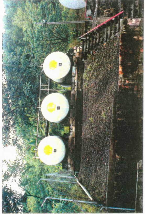
Photo 71: Fuel Tanks, Power Station
