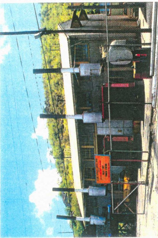
Photo 75: Vieux Fort Power Station
