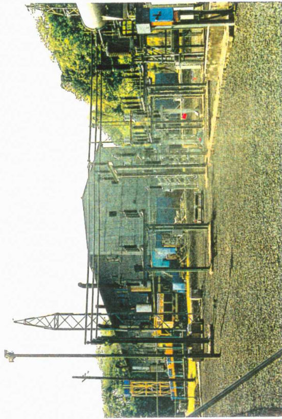
Photo 4: Union power station, on higher ground than the substation, was not affected by the flood. However, the generating facilities had to be shut down after the sub-station was flooded.
