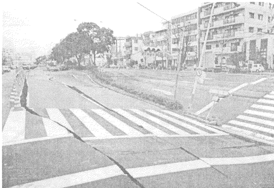
Photo 11 Artery Road Cut by Ground Failure Ground liquefaction made roads impassable Hyogo Prefectural Government
