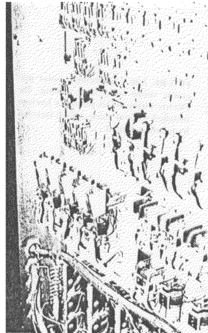
FIGURE 3.45. Motor control panels showing dynamically sensitive switches. This tall, slender panel is neither base anchored nor top braced.
