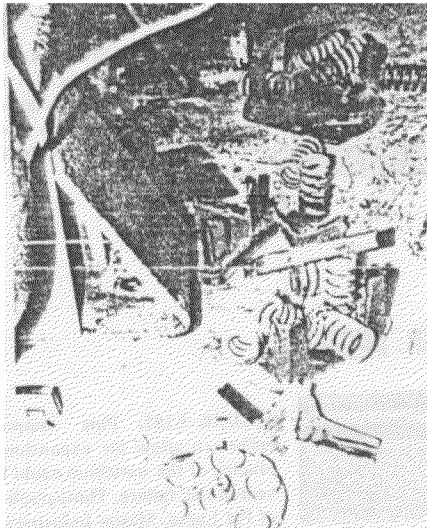
FIGURE 3.173. Collection of vibration isolators that failed as a result of not being provided with motion restraints. The vibration isolator housing should not be constructed of brittle materials. Photograph courtesy of Richard Miller and the National Science Foundation
