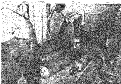
FIGURE 3.190. High-pressure gas cylinders that were supported by light-weight chains. The chains were not adequately anchored to the wall in the background. Photograph courtesy of Richard Miller and the National Science Foundation.
