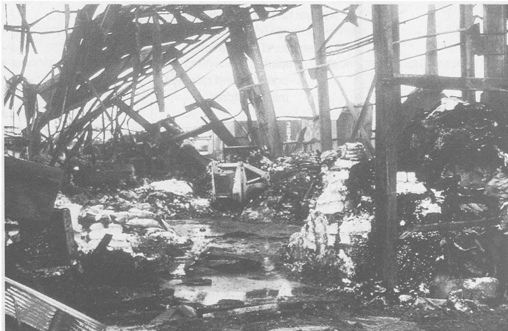
Consequences of fire in a factory, Melbourne, 1985. Photo : F. BALKAU
