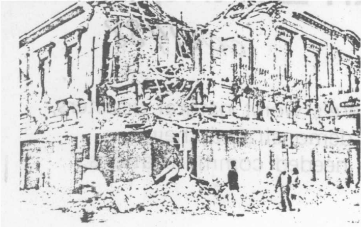
Three-story building in downtown Guatemala City bears mute testimony to the giant force that struck the city. (UPI photo)
